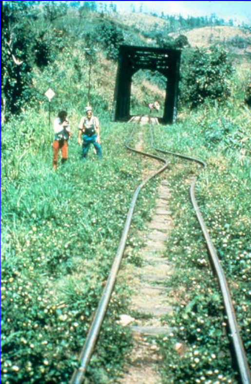
Railway track buckled by faulting. Guatemala 1976 (M = 7.5)
